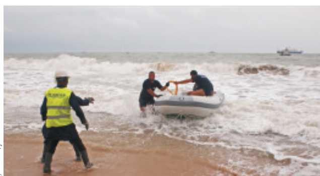
GLOI submarine cable landing in Lagos, Nigeria, Africa
